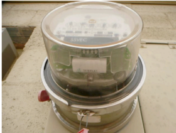
A General Electric meter with a PLC transmitter mounted on the bottom. The green circuit board can be seen. The Turtle logo on the white label identifies the meter as a PLC transmitter. The white label has a bar code on it, which is blanked out for privacy.
