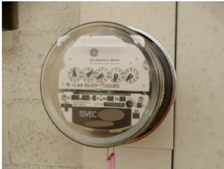
Analog meter with hidden PLC transmitter. The serial number has been blanked out to protect privacy.
